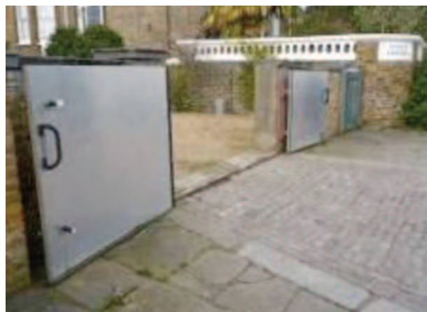
Above: Example of a flood gate installed to a communal car parking area
